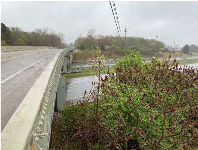
FIGURE 4. Photo looking east on the south side of the Howell Road bridge over US-127.
