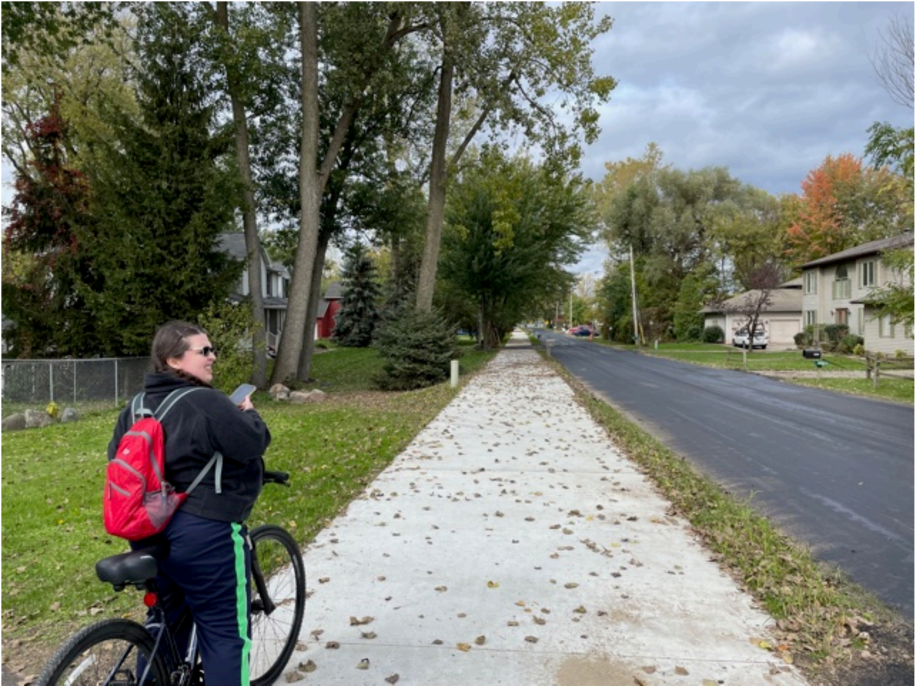
Part of new widened sidewalk MSU to Lake Lansing Trail connector to Lake Lansing South Park
