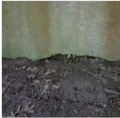
Exposed sheet piling at West Abutment (no riprap)
