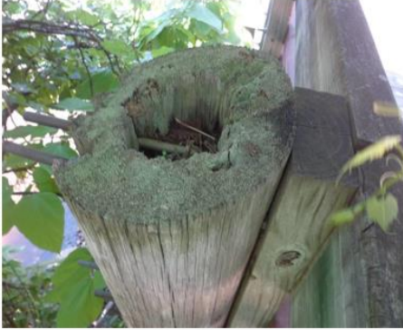
Typical rot on pier cap
