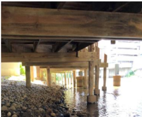
Weathered piles in waterway (typical)
