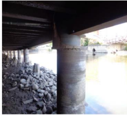
Typical outside pier column with misalignment
