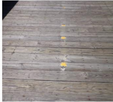
Typical walkway decking
