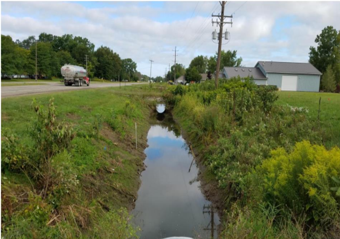
Photo 6. Typical Ditch to be Filled and Replaced with Underground Stormwater, Looking North
