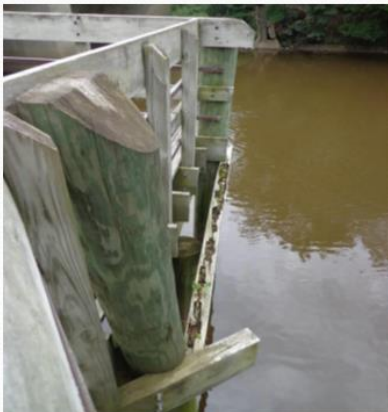
Rot and mold on Bracing at Pier 19
