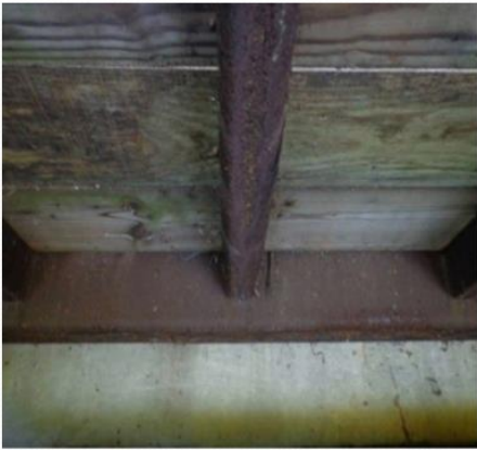
Bulging beam 2S at East Abutment
