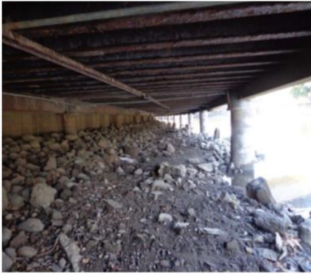
Typical condition of beams (section loss)
