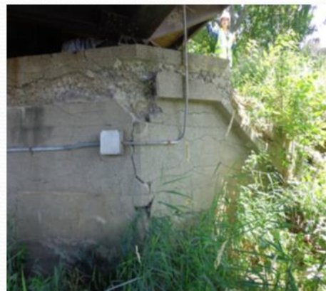
Damaged southeast wingwall
