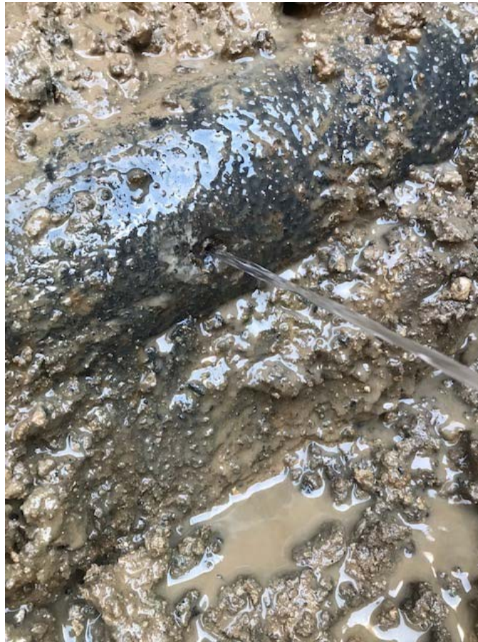
LEAK IN MAIN SNOW MAKING LINE
