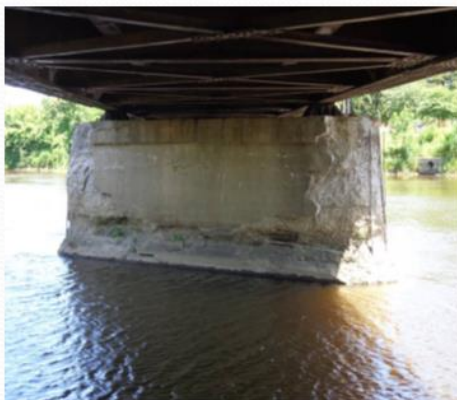
Damaged west pier
