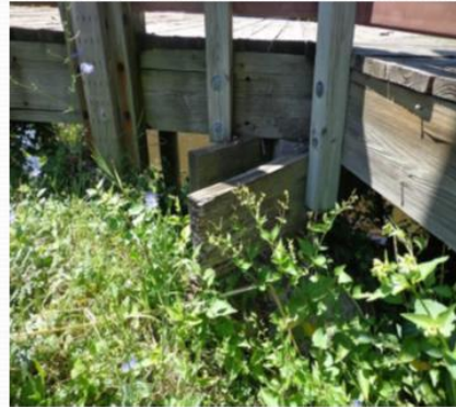
Typical rot on pier
